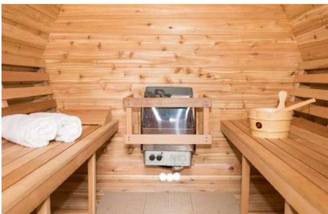
Inlet under electric heater on Back wall
