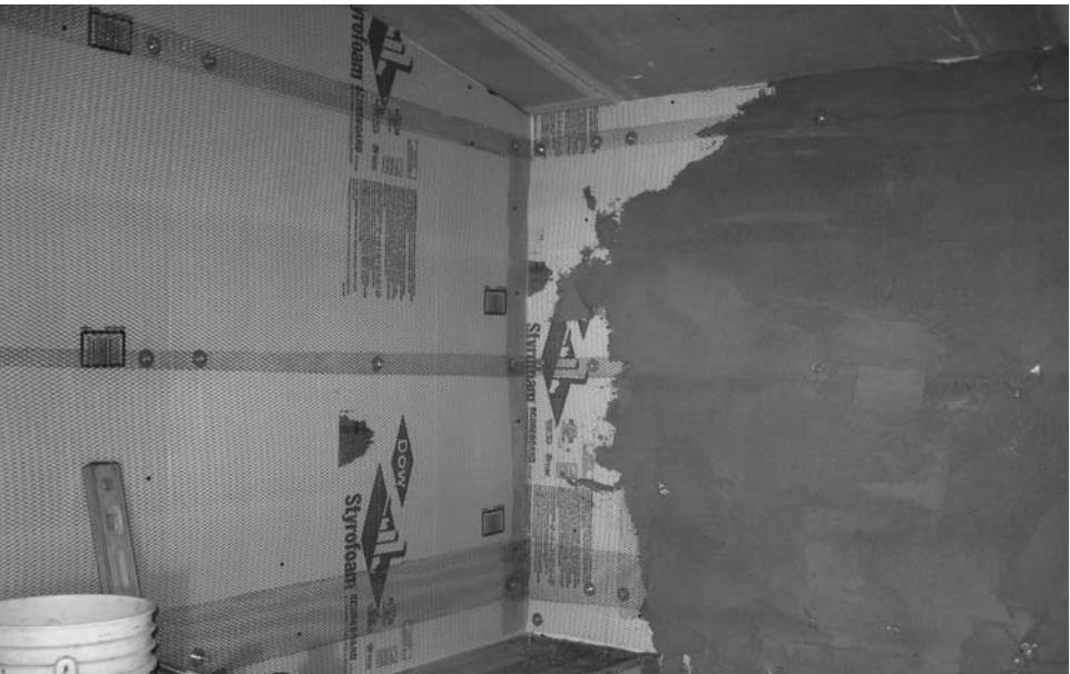
Wall partially finished with scratch coat of LATICRETE® 226 Thick Bed Mortar and LATICRETE 3701 Mortar Admix.
