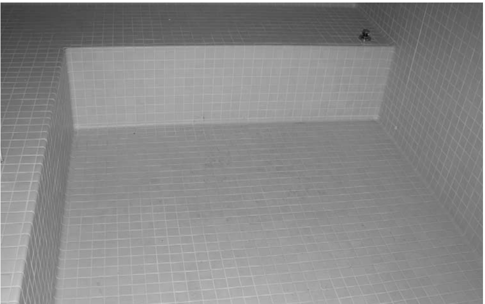
Finished floor installation of tile. Floor and seats are sloped 1/4 " per foot (6 mm per 300 mm) to the drain.
