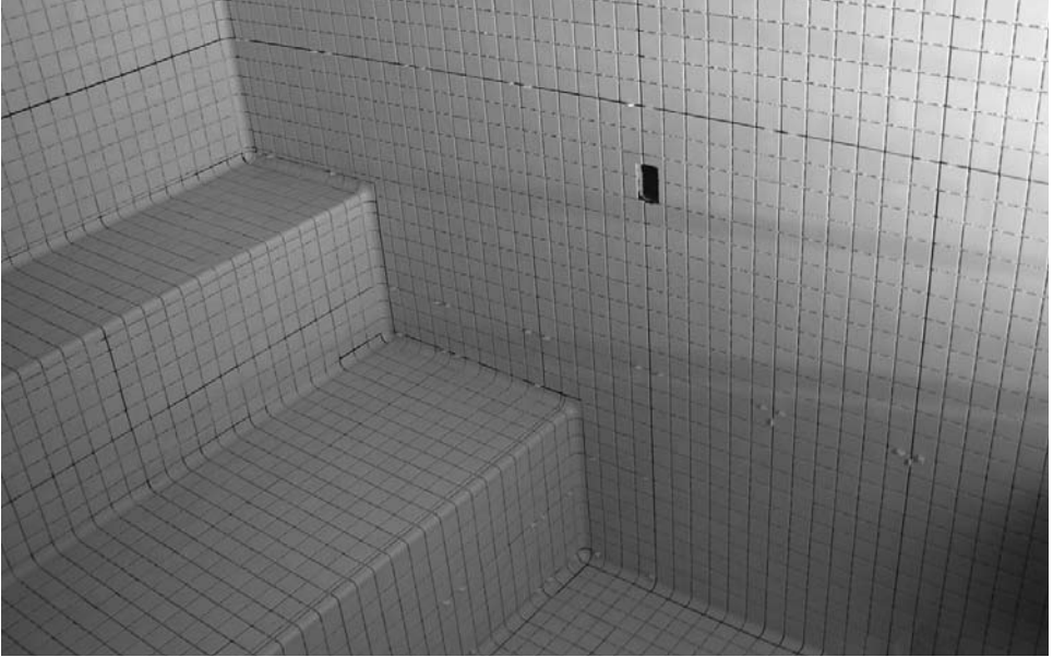
Finished installation of 2" x 2" (5 cm x 5 cm) vitreous tile using LATICRETE® 254 Platinum. Notice the cut-out for the emergency call switch.
