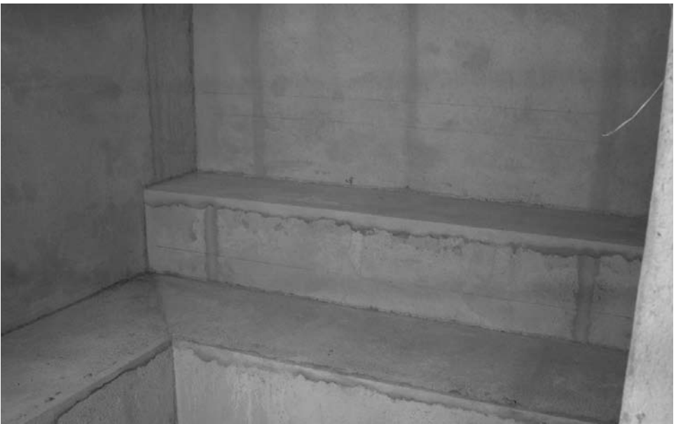
The steam room seats after the installation of the LATICRETE® 3701 Mortar Admix and LATICRETE 226 Thick Bed Mortar.
