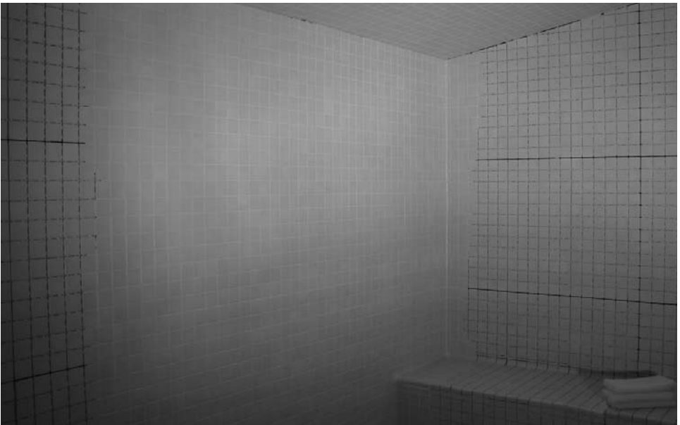
Installation of LATICRETE 1500 Sanded Grout mixed with LATICRETE 1776 Grout Enhancer on ceiling, walls and seat.
