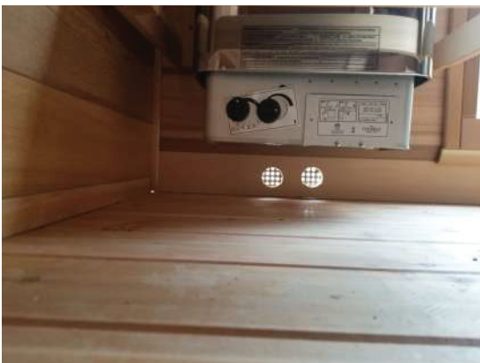
Inlet under electric heater on Back wall
