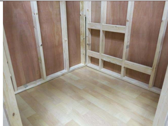
Photo 01. Notice location of bench support blocking.
