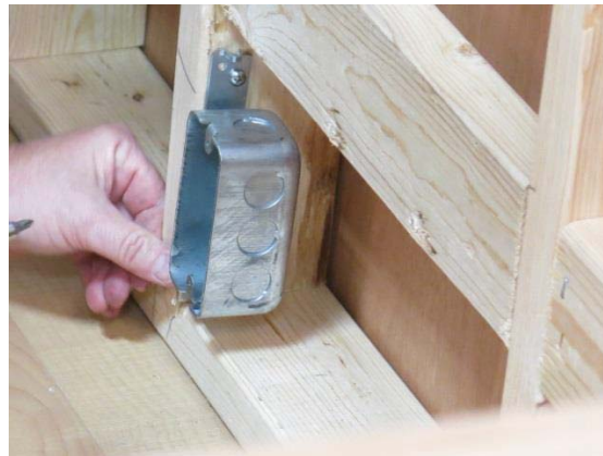
Photo 04. Mount just above bottom framing plate so all boxes will be below the lower bench. Make sure the box is positioned to be flush with your finished wall surface.
