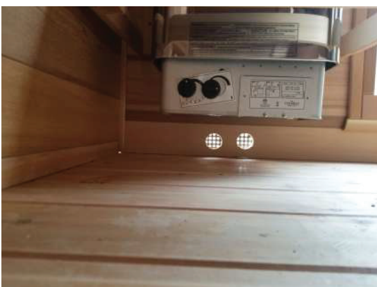
Inlet under electric heater on Back wall
